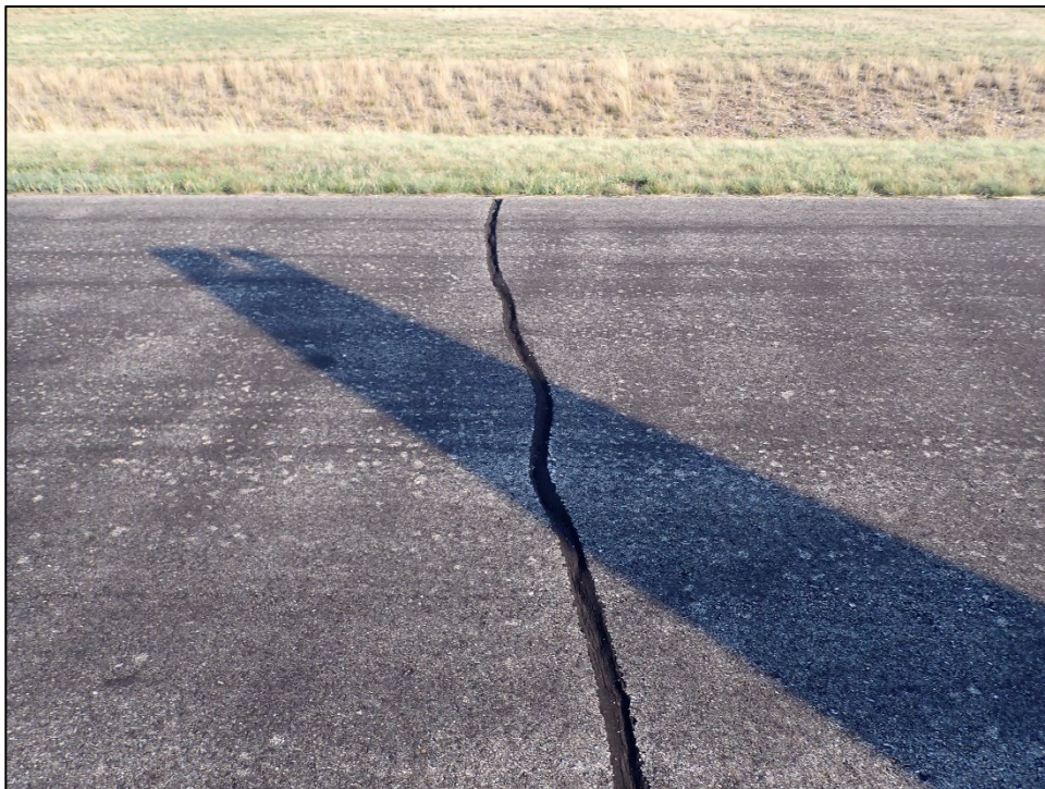
AP-11-15: L&T Cracking
