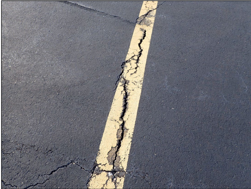
AP-11-10: L&T Cracking
